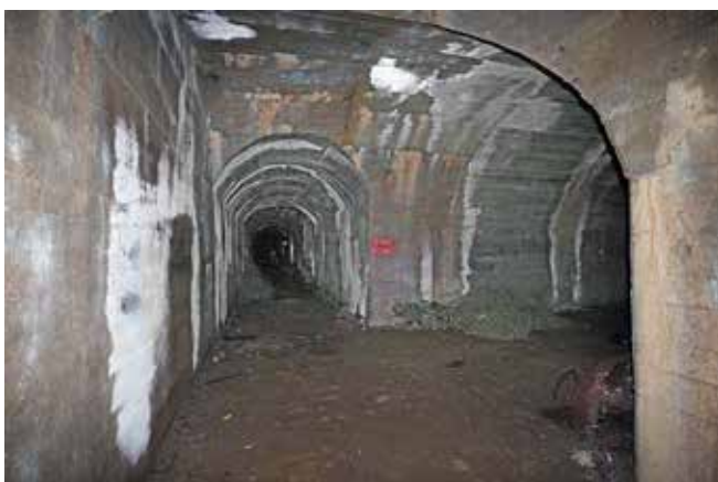
Looking north along the storage tunnel; the first of the storage bays is seen on the right. Rubble from the collapsed unlined storage bay on the left is seen straight ahead. The 'fire point' sign on the wall was painted by the liberation forces in 1945 during clearance of the tunnels
